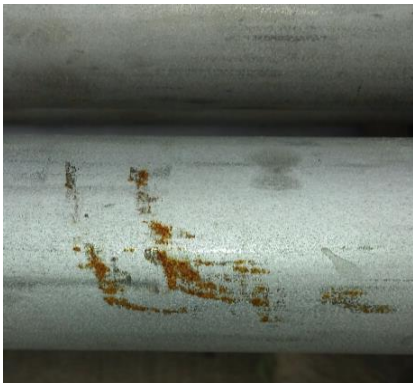
Figure A: Pipe with embedded rust.
